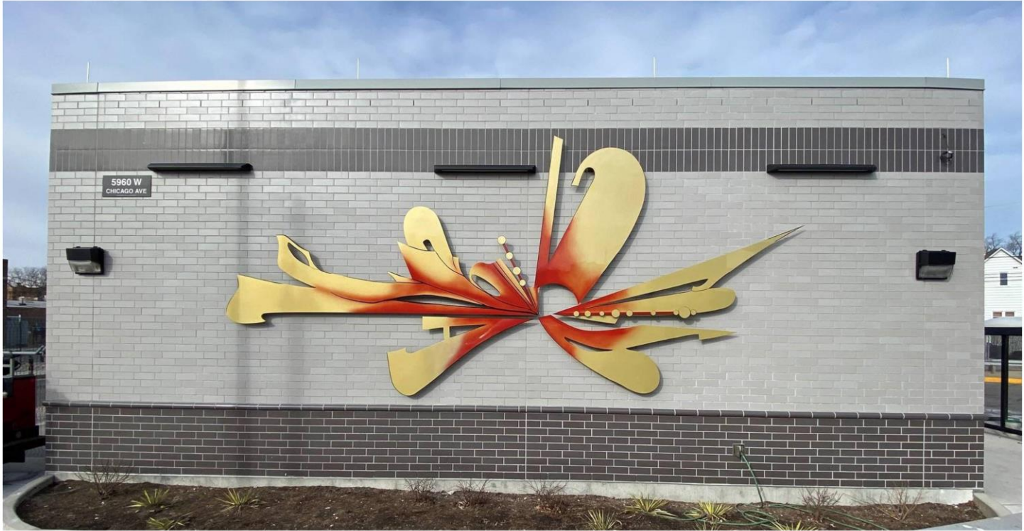
Electric Substation for E Bus Charging with Public Artwork At Chicago and Austin Bus Terminal
