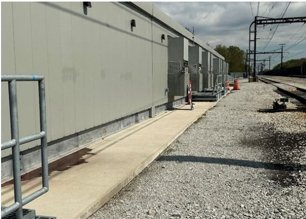
New Matteson Substation.
