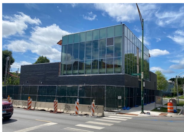
New Barry Substation
