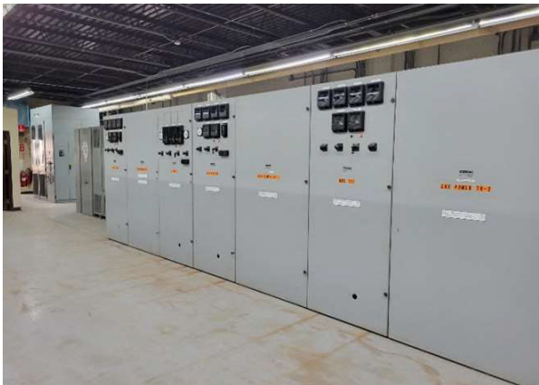
Switchgear inside the existing Jackson Substation.
